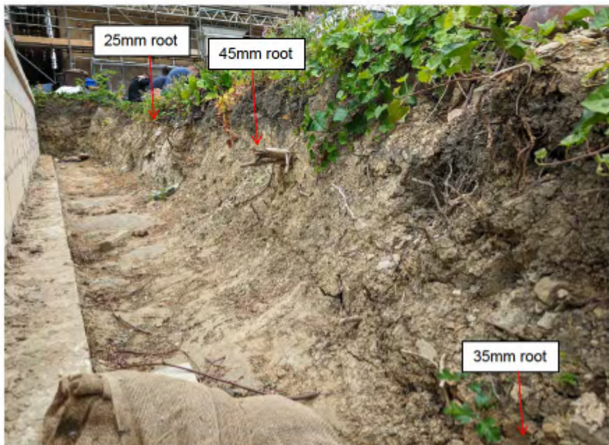
Major roots identified within excavation of 4 Bromgrove Road retaining wall.
