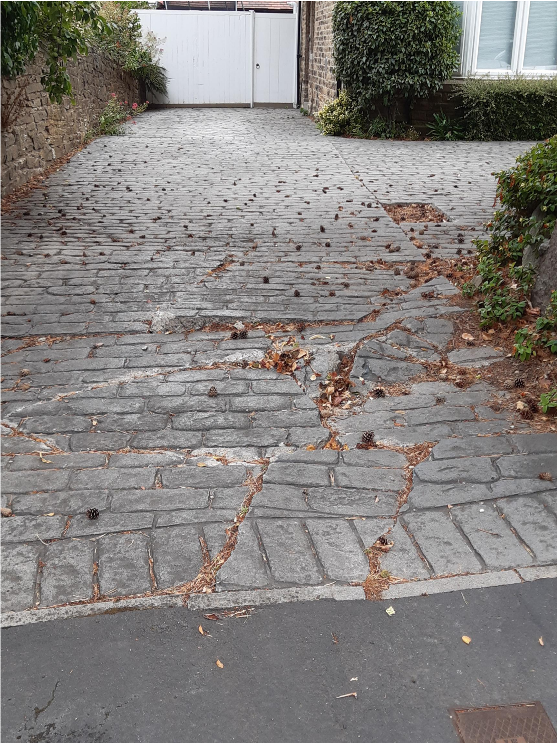
Image of damage to drive.
